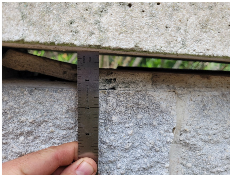
Figure 2: View of crack / separation in the privacy wall.
