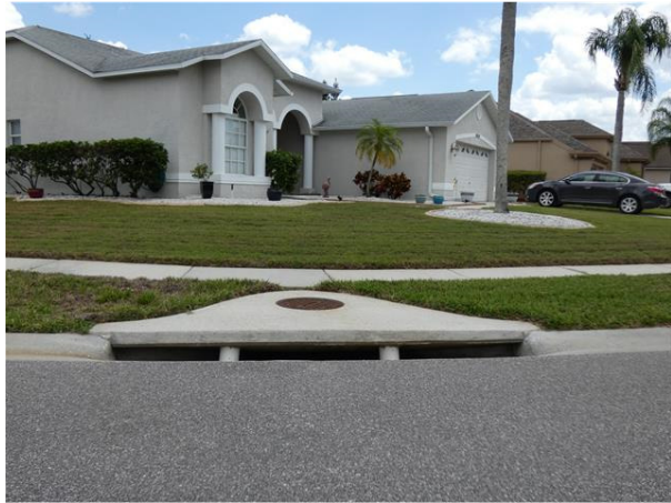
Stormwater Drainage Curb Inlet
